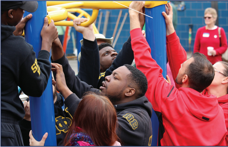
Recess at Sheridan Preparatory Academy will be a lot more fun thanks to a new playground built on Oct. 8 with help from a grant and the community.
