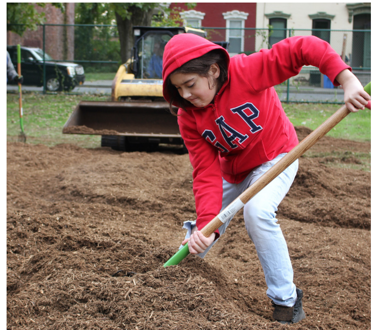
If you've ever wondered how long it takes to build a new playground, Giffen Memorial Elementary School has the answer: two days! The project was completed Oct. 25-26 thanks to help from St. Peter's Health Partners, hard-working staff and, most importantly, the students who will enjoy the play structures for years to come. Giffen sixth-grader Juan Padua was one of many students who helped with the heavy lifting Oct. 26.
